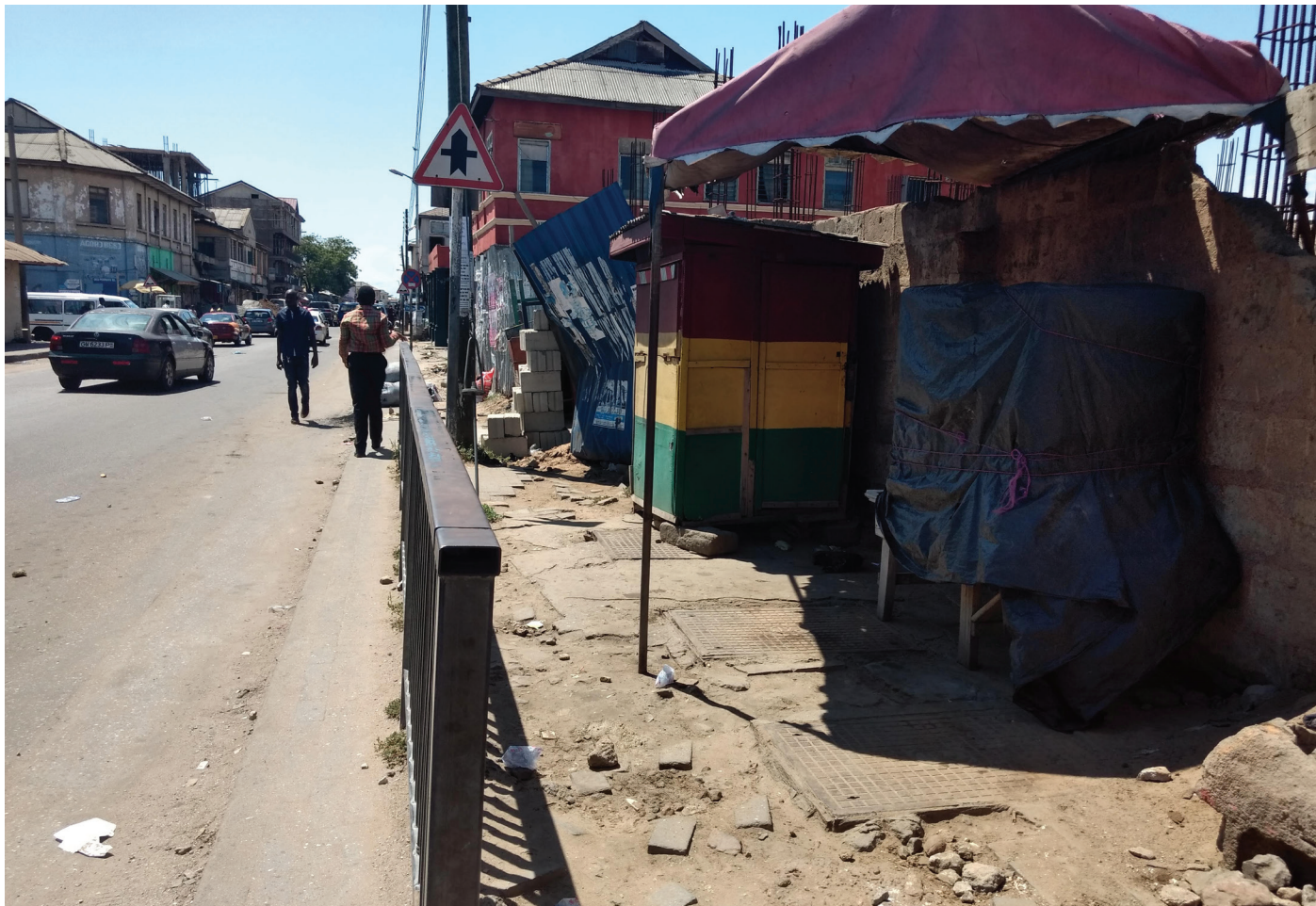
Looking west along Asafoatse Nettey Road. The sidewalk obstructions, including the guardrails, cause pedestrians to walk in the streets.
